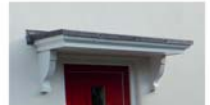
Traditionally Dartmoor townscapes feature very low porches and canopies. However, consultation has highlighted that there is a strong preference for some external protection so canopies will be incorporated to all dwellings.
